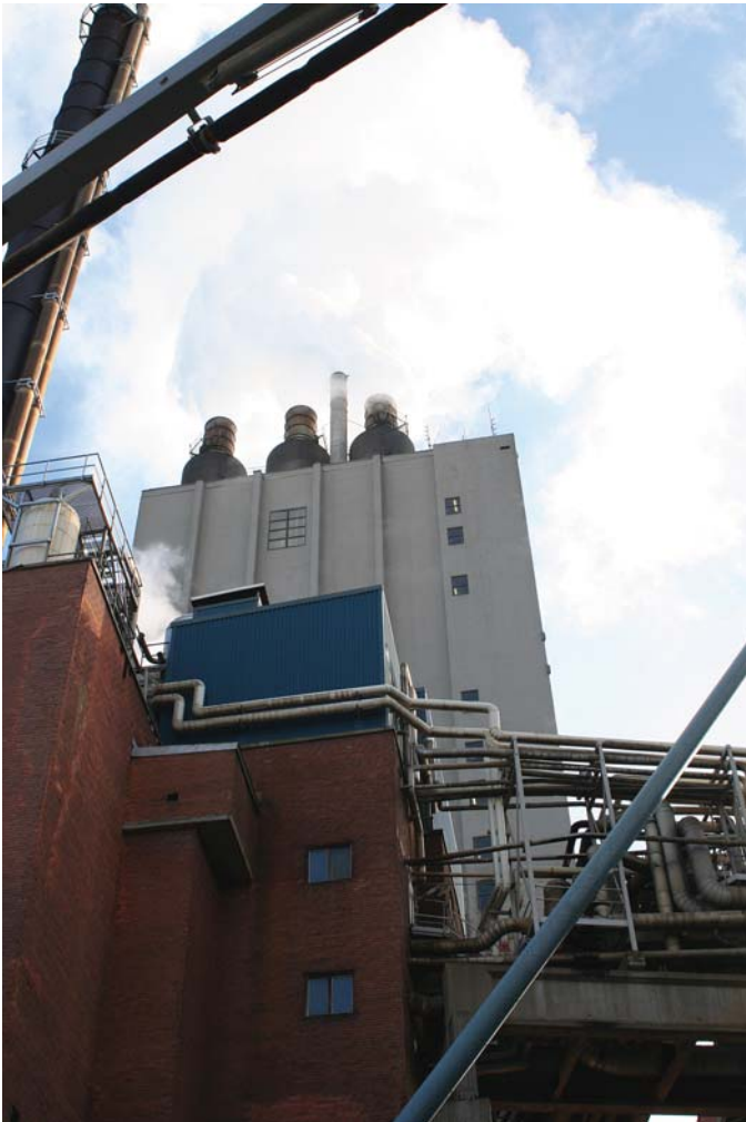
A gas cleaner installed in 2008 has reduced nitrous oxide emissions to air from burning sludge by 200 tonnes per year.
