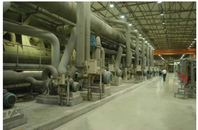
The de-inking cells and giro cleaners at the Aylesford Newsprinters in the UK, which produces recycled newspaper stock.
