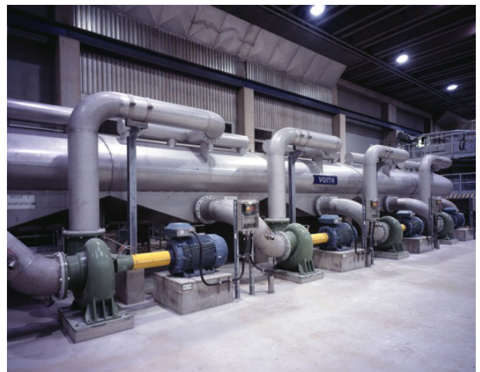
A typical flotation deinking machine. Image courtesy of Voith Paper.
