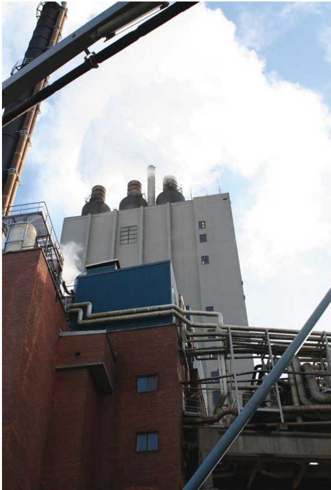
A gas cleaner installed in 2008 has reduced nitrous oxide emissions to air from burning sludge by 200 tonnes per year.
