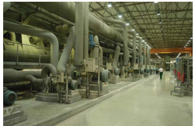
The de-inking cells and giro cleaners at the Aylesford Newsprinters in the UK, which produces recycled newspaper stock.
